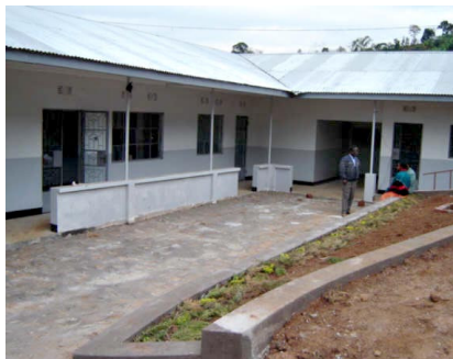
New complex: The almost-completed wing of the Shighatini health care center, a surgery suite and exam rooms, August 2006
