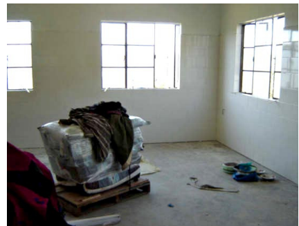
Operating room: Surgical equipment being unloaded in the new surgery suite, September 2006
